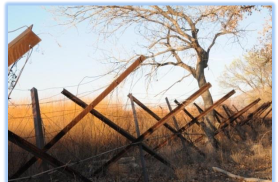
Kelmer jetty jacks were installed along the banks and through the floodplain to stabilize and prevent lateral movement of the river channel.
