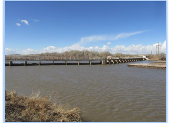
The Isleta diversion dam provides irrigation water for the MRGCD Belen Division.
