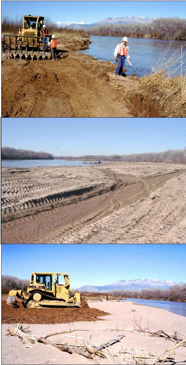
Figure 7. Mechanical manipulation on the AOP site prior to flooding: a) all introduced Russian olive was root plowed; b) the bar area adjacent to the river was lowered 0.6 m and channels and bars excavated; and c) the sediments from the lowering were deposited at the distal end of the bar.
