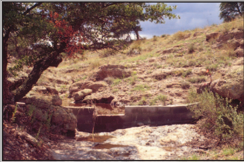
The sediment dam at Cascabel Watershed, New Mexico, is used to measure sediment production related to land management activities. (Photo by Gerald Gottfried)
