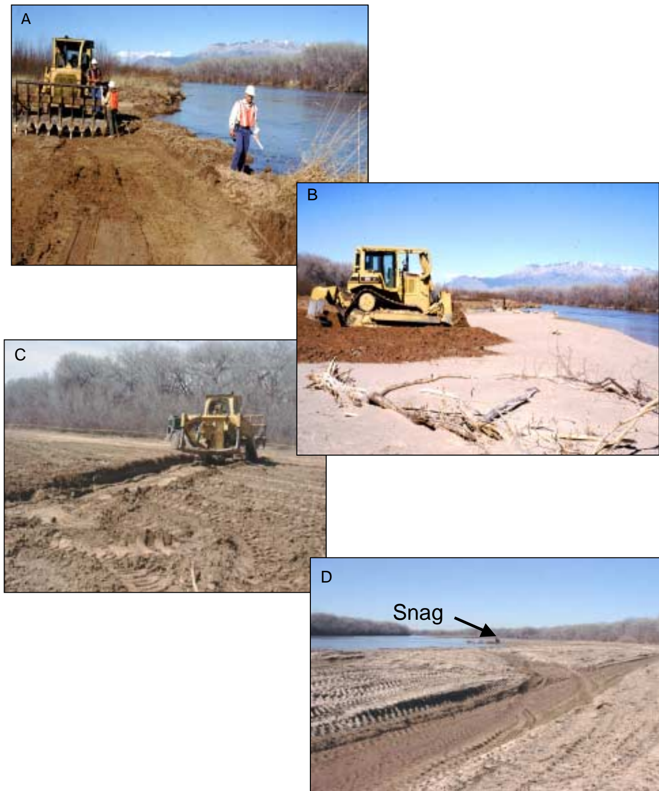
Figure 5. AOP site treatment was begun in March 1998 with the clearing of a Russian olive stand and the lowering of the bar by approximately 0.66 m (two ft) (A). Materials were moved onto an adjacent sandbar downstream (B). Channels and low-lying islands were excavated into the new bar to create microhabitats for cottonwood regeneration (C and D).
